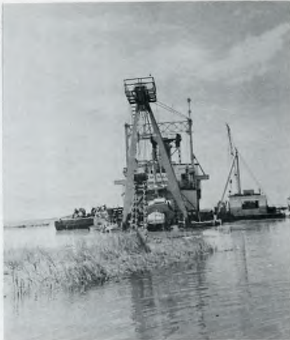
The " Business End " of the 27-inch Hydraulic Dredge " CARTAGENA " boring into the depths of the St. Clair River at Southeast Bend. The total amount of material removed, 22,000,000 cubic yards of sand and soft clay would cover the entire area of Belle Isle for a depth of 15 Feet. #298-60
