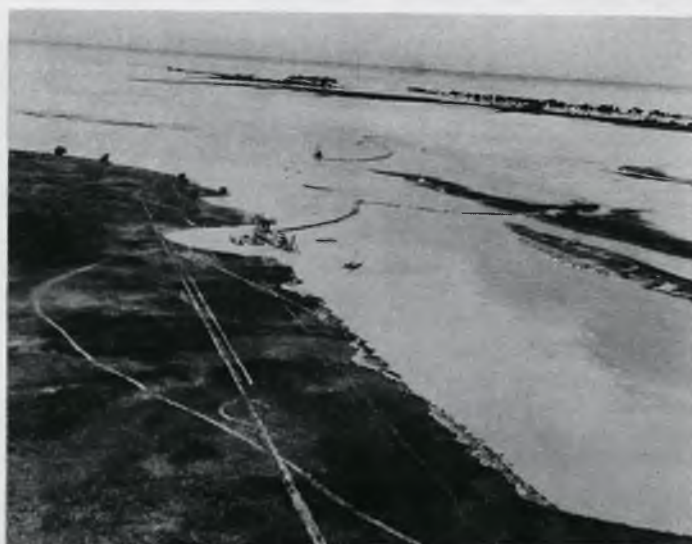
Aerial photograph looking downstream on the Southeast Bend Cutoff channel, 700 feet wide, five miles long and 27 feet deep, which will replace the hazardous Southeast Bend channel. The 27 inch pipeline dredge CARTAGENA in foreground, and the 20 inch dredge SHUNIAH are busily at work.
