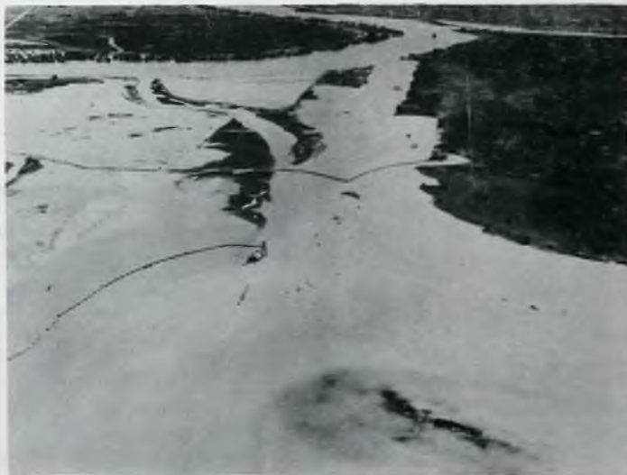
Aerial Photograph looking Northeast from Lake St. Clair, of the Hydraulic Dredging Work being performed on the New Cutoff Channel, Lower St. Clair River. The Dredges SHUNIAH and CARTAGENA are busy scooping out material for this new passage. # 326-60
