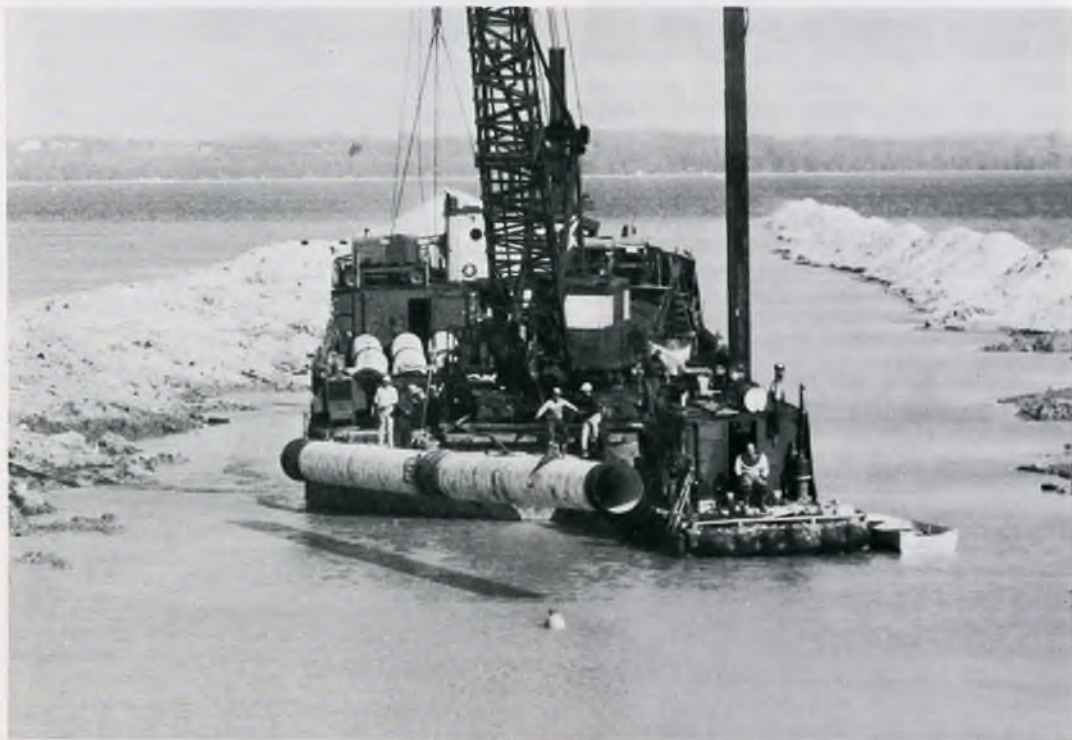
The J.B.II laying 48" pipe in Grand Traverse Bay. The tending tug is Bultema's South Haven.
