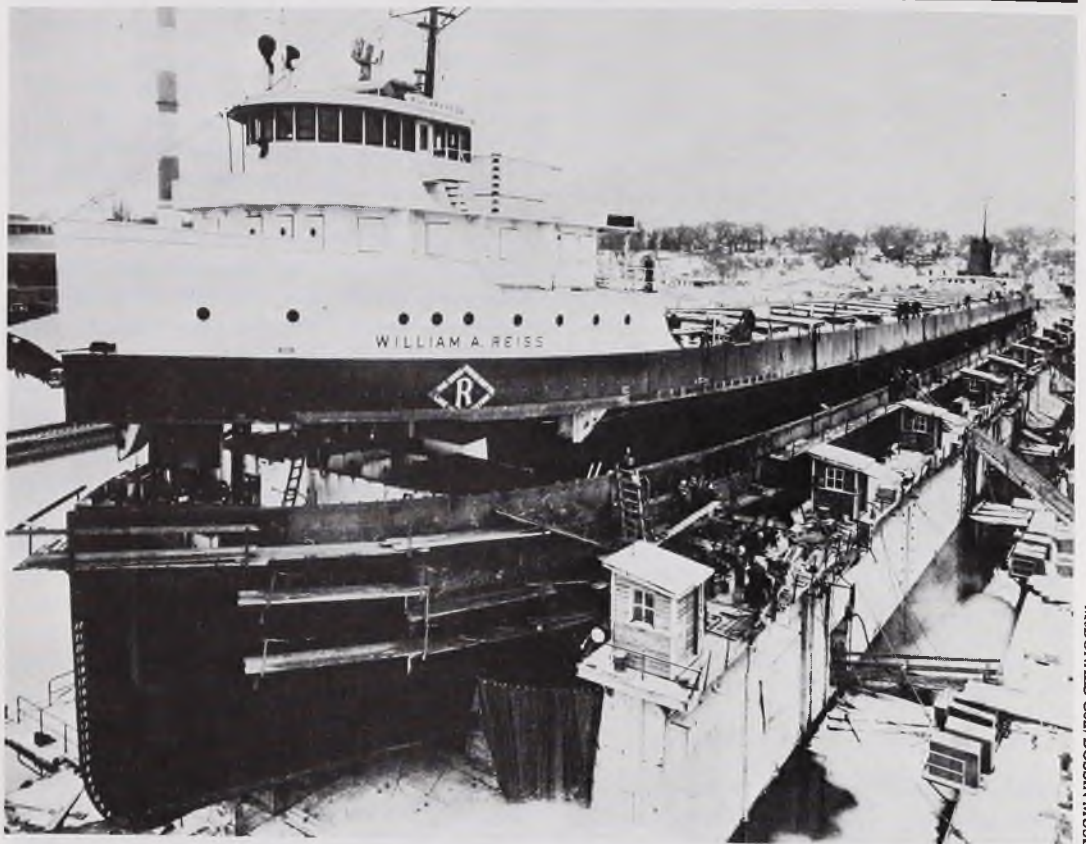
Major surgery, this view in the Manitowoc dry dock in the winter of 1962-63, when the WILLIAM A. REISS had her deck jacked up 7'-6" in a unique deepening procedure. Specially designed hydraulic jacks were used to raise the deck in a single unit.
