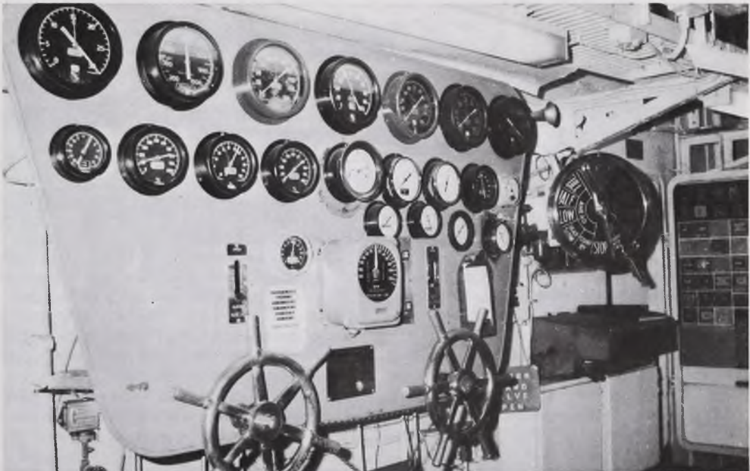
Although her engine room remains little changed since being built, the subsequent modernization still leaves the original turbines and boilers intact.
