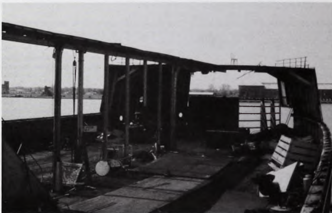
Top: Purvis Marine cutting down the CHIEF WAWATAM to a barge on April 9, 1989. Bottom: Workers clear out the inside cabins and tracks on the CHIEF. The notch has been cut in the stern to accommodate a tug.
