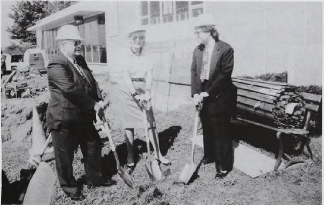
The groundbreaking was held on July 24th. From left to right are Al Jackman, president of the GLMI, Mrs. Barbara Wrigley, president of the Historic Commission of Detroit and Steve Robinson of the Erwin Robinson Company, donators of the WCF pilothouse.
