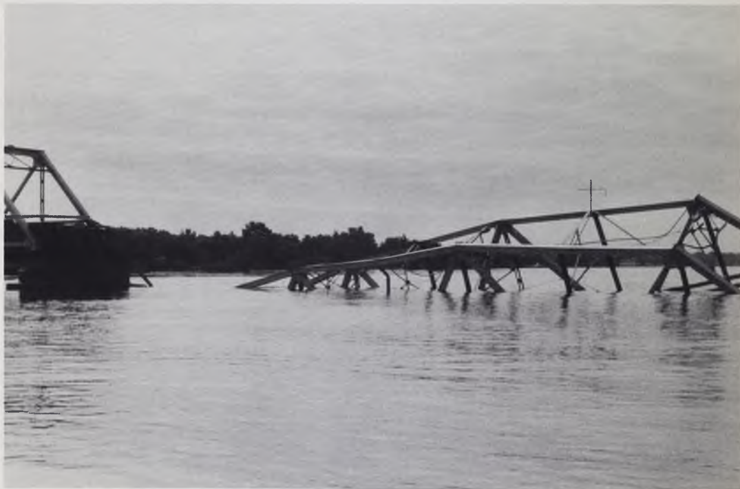
Salvage crews removed the sunken span of the Grosse Ile Toll Bridge and dismantled it at McLouth Steel's dock.
