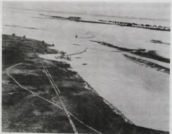
Aerial photograph looking downstream on the Southeast Bend Cutoff channel, 700 feet wide, five miles long and 27 feet deep, which will replace the hazardous Southeast Bend channel. The 27 inch pipeline dredge CARTEGENA in foreground, and the 20 inch dredge SHUNIAH are busily at work.
