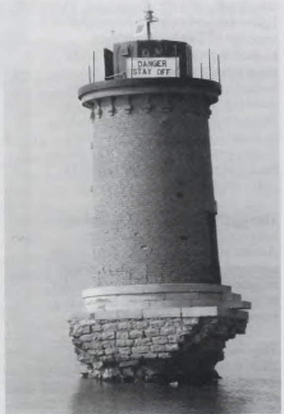
View of Front Light, 1988. Note the solar-powered navigation beacon installed by the Coast Guard and the deterioration of the base.
