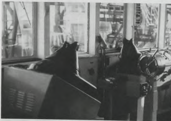
Radar units still intact and in working condition.
